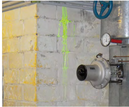
Detection of a leaky water-carrying pipe in a building by passing in Uranin and performing a subsequent UV inspection.
