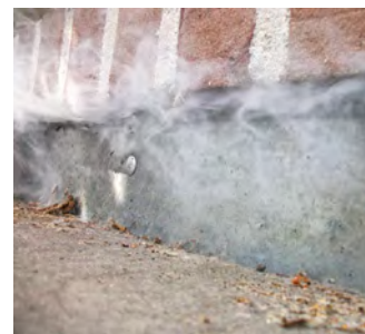
Evidence of defective sealing of the wall connection above an underground garage.
