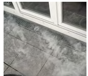
Defective sealing of a roof-top terrace.
