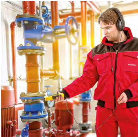
Signs of wear at pumps and other processing machines can be detected at an early stage using the structure-borne sound probe.
