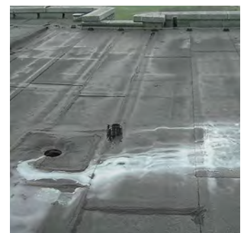
Typical Luminat applications are for instance examinations of flat roofs for detecting a sealing flaw by means of dye testing.
