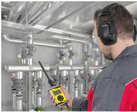
Using the directional sound probe, leaks at exposed lines can be located precisely.
